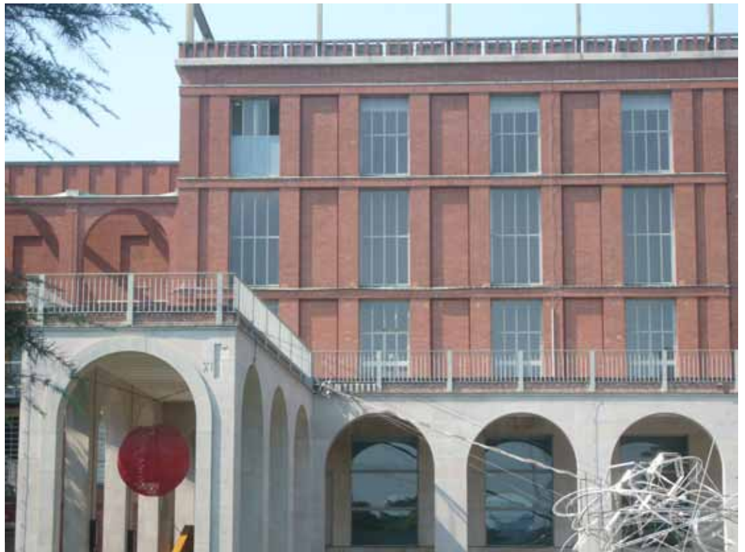
Palazzo dell 'Arte Terugliggend metselwerk met extra schaduwrand / Recessed brickwork surfaces with border of shadow
