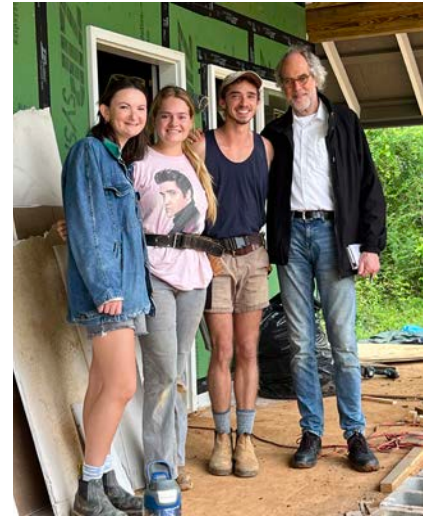
Three Rural Studio students with Jan Timmers in front of a double house under construction by the students. The houses will be occupied by homeless families as a transition to a permanent home.
